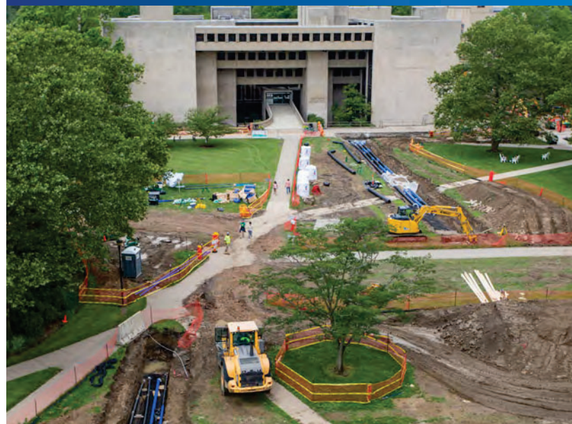
Aerial view of Oberlin College and Conservatory's new heating and cooling distribution piping, installed as part of the new carbon-free district energy system. Photo credit: Yvonne Gay Fowler
